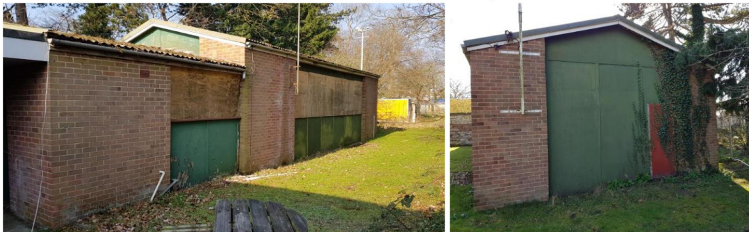
Photos 12 and 13: The Pine Hall constructed in 1975 (Photo taken February 2018). Demolition and landscape is proposed as part of a comprehensive scheme of landscape enhancement.
